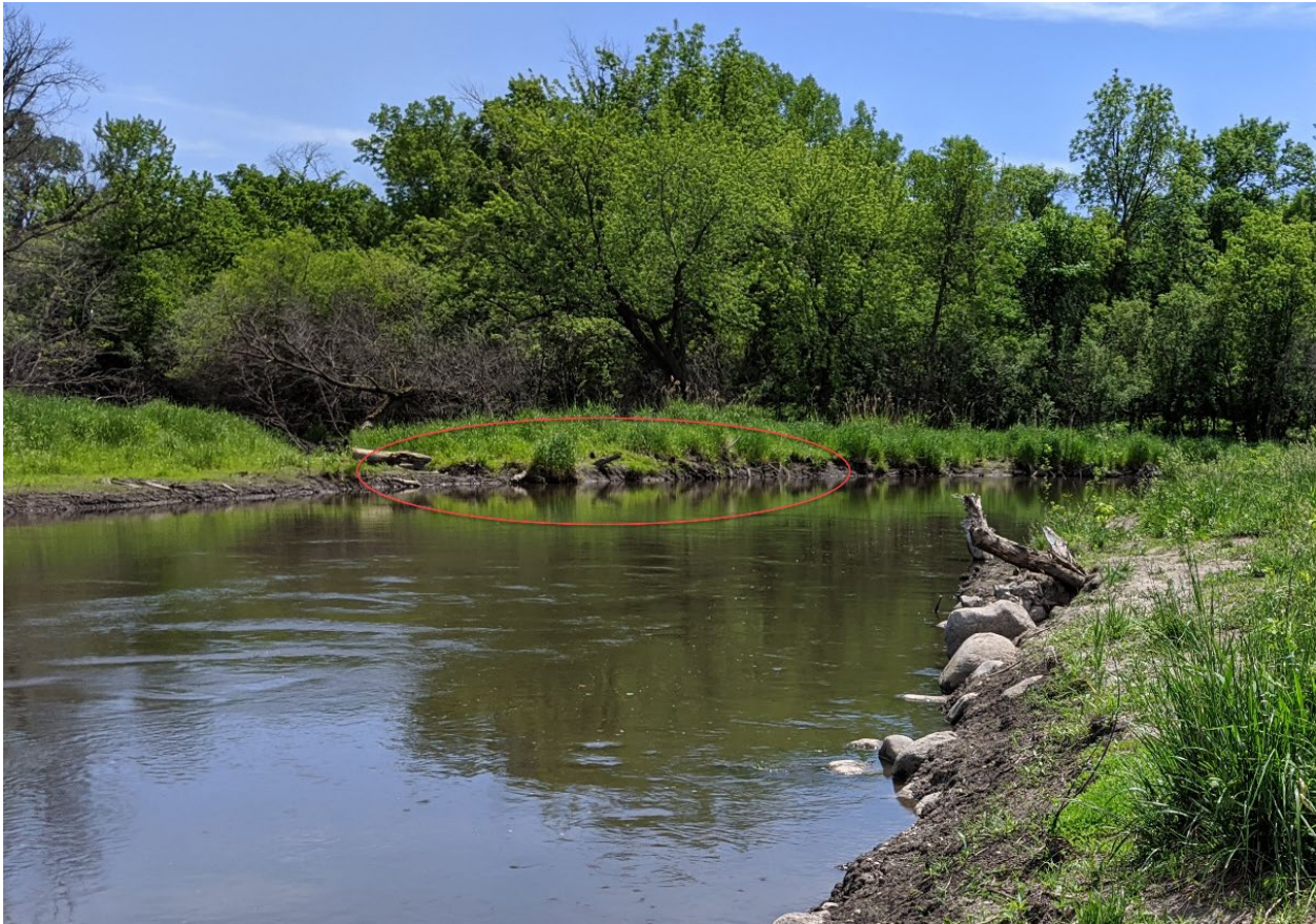
Figure 6-13: Plug of Cut-Off Channel using Toe Wood-Sod Mat on the Pomme de Terre River in Minnesota
