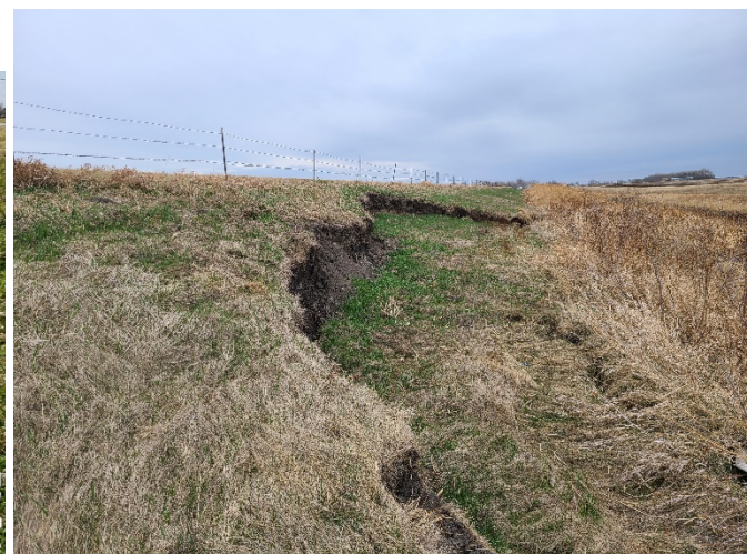
Figure 2. Existing slope sloughing (looking east)
