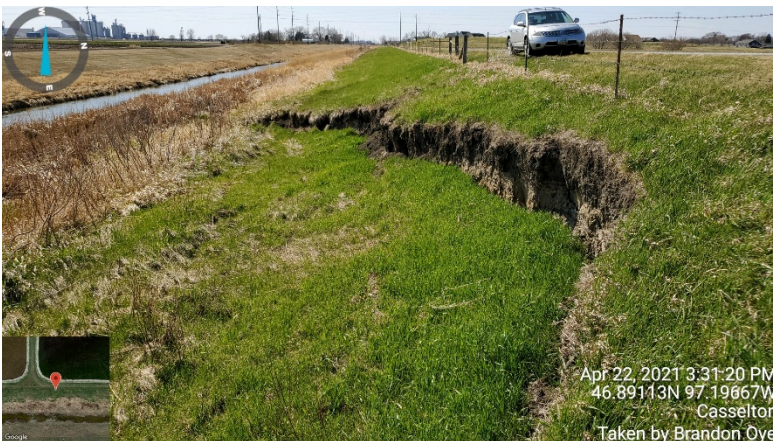
Figure 1. Existing slope sloughing (looking west)
