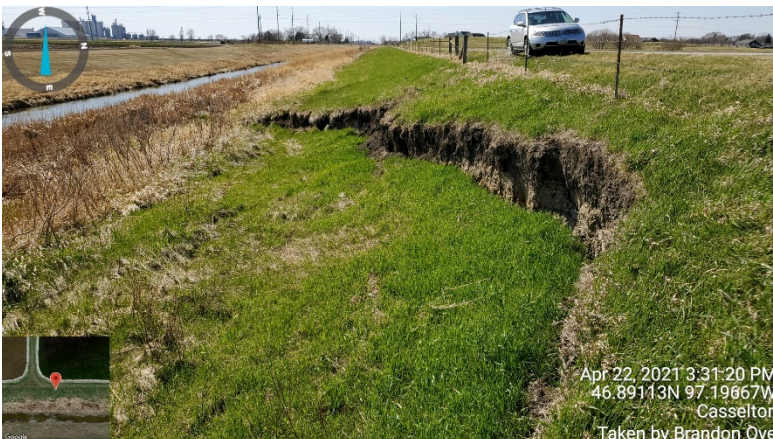
Figure 1. Existing slope sloughing (looking west)
