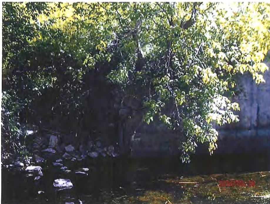
Photo #8 – Bank erosion and tree growth at the downstream end of the south spillway wall.
