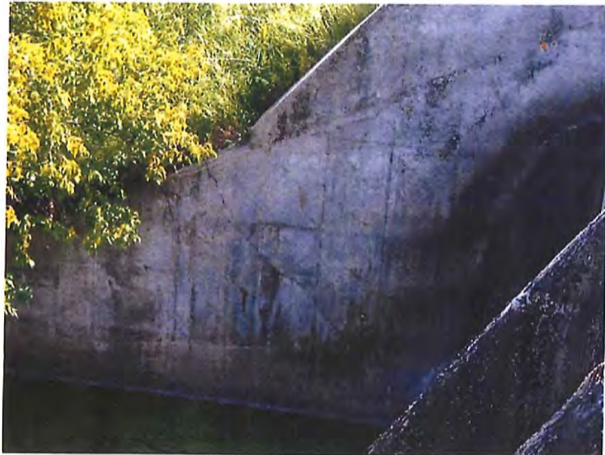
Photo #6 – Fine cracks on south wall of spillway.
