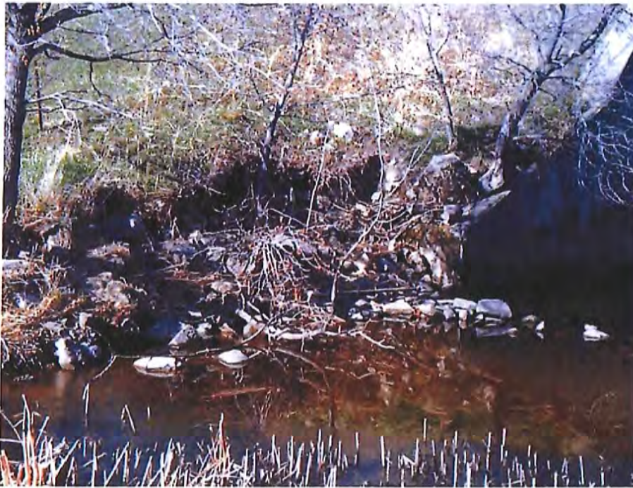
Photo #9 – Bank erosion and tree growth at the downstream end of the south spillway wall (April 2012 photo).
