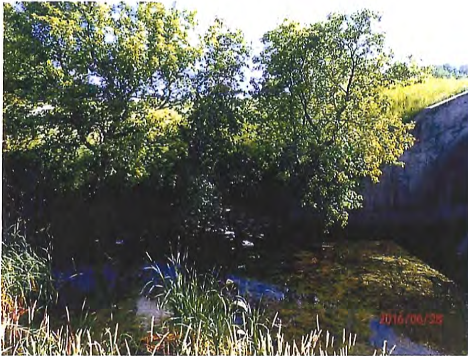
Photo #7 – Large trees growing at the toe of the embankment on the south side of the spillway.
