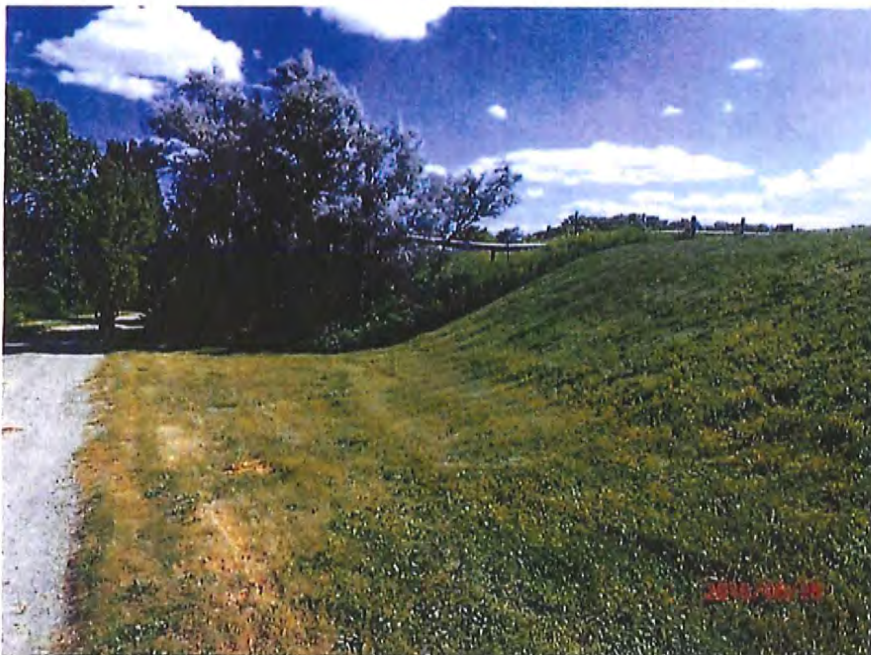
Photo #4 – Downstream slope, looking south. Note the large trees growing at the toe of the embankment.
