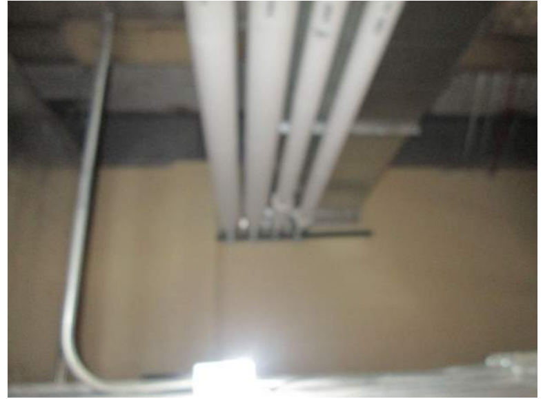
Chiller piping and large ducts through west wall mechanical room
