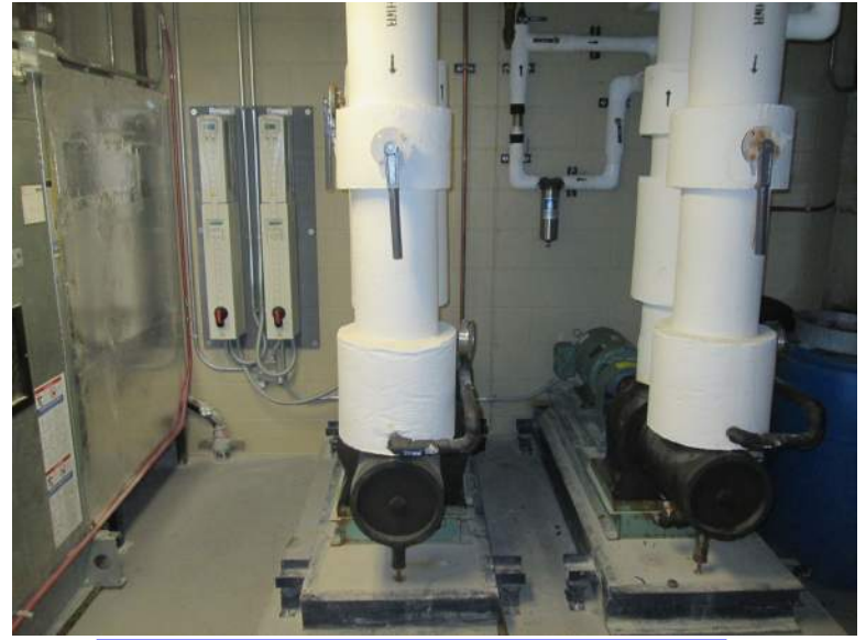
South wall mechanical room @ pumps
