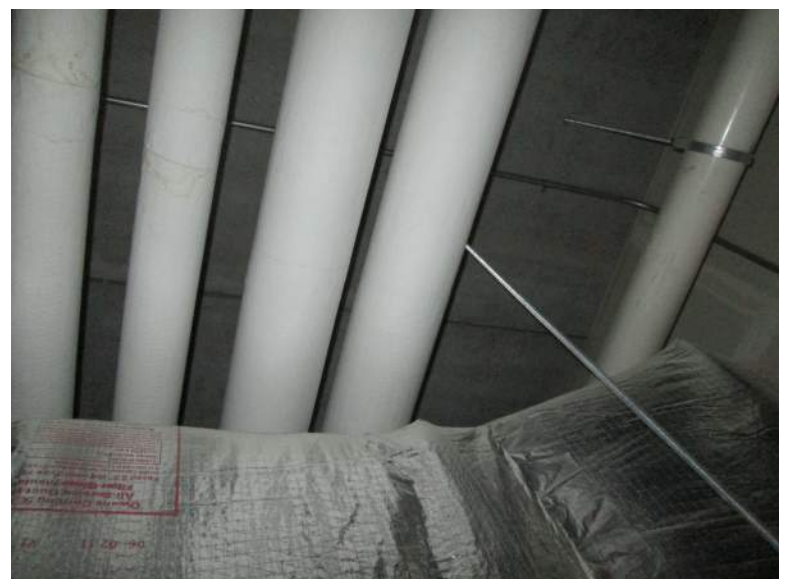
Chiller piping above IT cubicles
