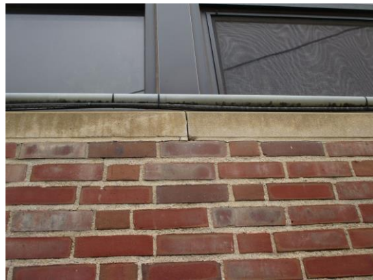
A10: Window sill.
