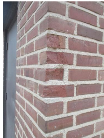
A12: Damaged brick at courtyard
