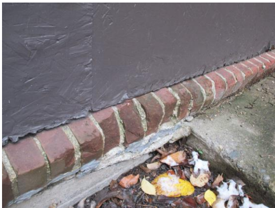
A9: Window Sill
