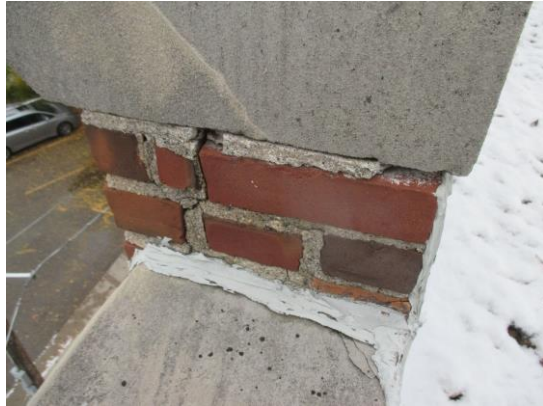
A2: Notch in parapet.
