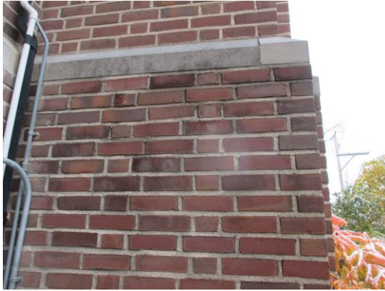
A7: Deteriorated mortar joints
