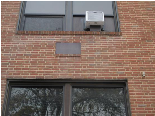
A53: Window A/C unit
