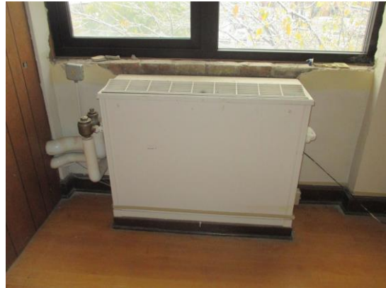
A48: Unfinished sill at replaced window
