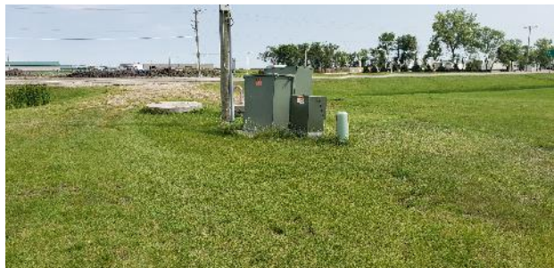
Existing Lift Station
