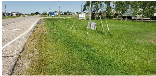
Power Pole and guy wires south of Knutson Street
