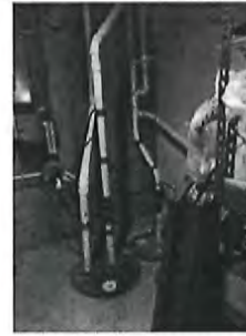
Basement Mech Room
