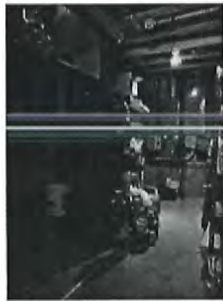
Basement Mech Room
