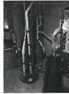
Basement Mech Room
