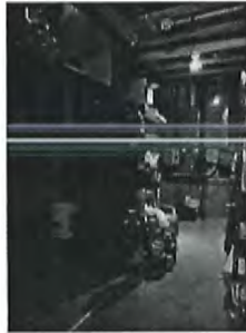
Basement Mech Room
