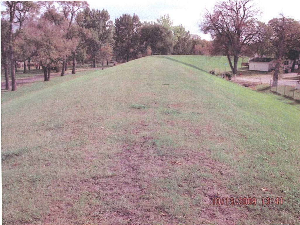
Federally Constructed Levee at 6 th Ave. S. and 3 rd St. S., Fargo, ND Example as will be discussed for Oxbow, ND at the January 8-10 Public Meetings Height of Levee Shown: 15 Feet Crown Width of Levee Shown: 10 Feet Side Slopes of Levee Shown: 1V:3H
