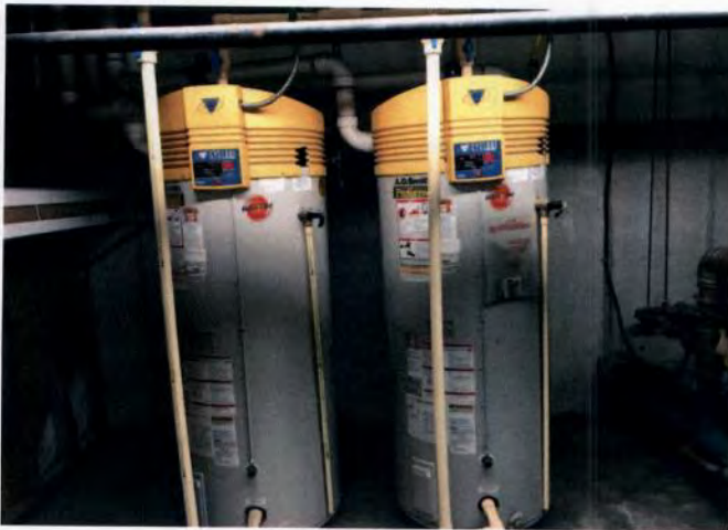
Hot Water Heaters
