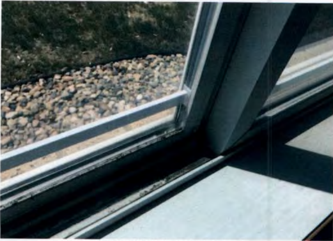
Typical Window Condition
