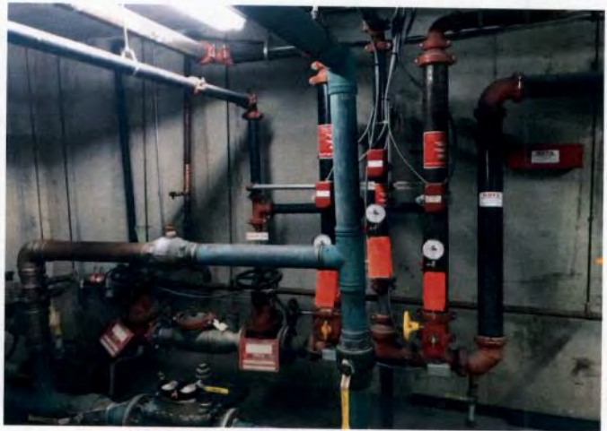
Water Main and Fire Sprinkler Risers
