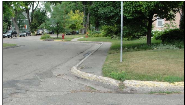
Sidewalk without curb cut, Moorhead
